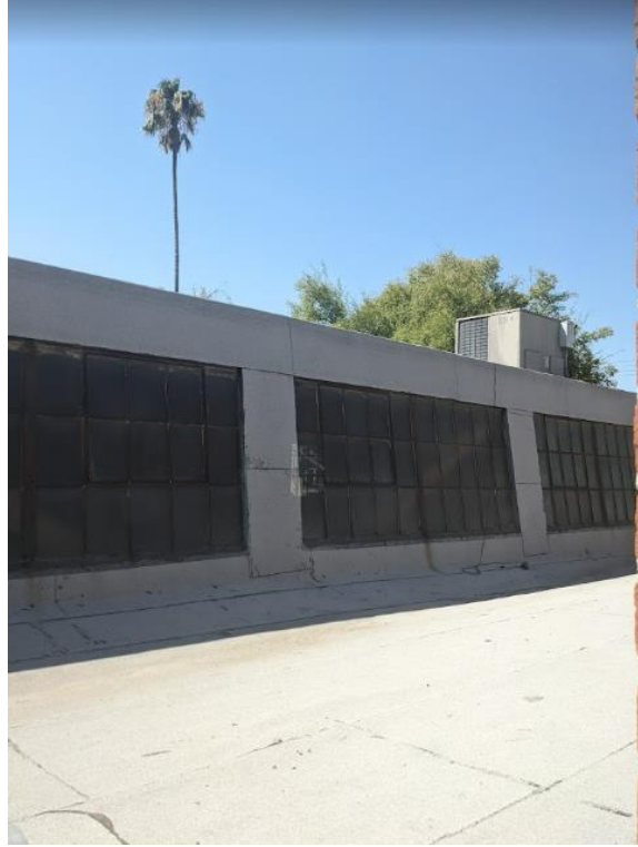
Figure 17. Windows, Main Factory Space (facing south from second-floor offices) SOURCE: Sapphos Environmental, Inc., 2022
