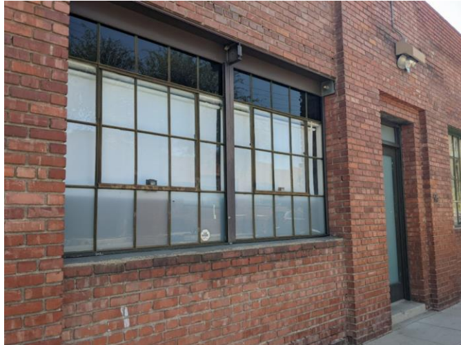
Figure 15B. Western Façade (detail showing steel sash windows and door) SOURCE: Sapphos Environmental, Inc., 2022
